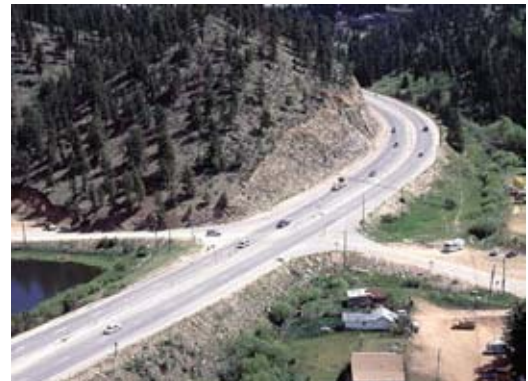
Site of Shaffer's crossing interchange and wildlife crossing at Elk Creek Road, which will run under US 285. Photo McGraw-Hill Construction
